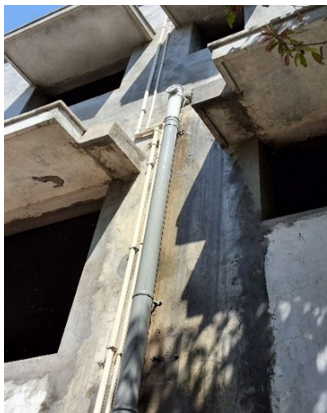
Fig 13: Improper packing of drain outlets in walls and slab lead to leakage of overflown water to the below structure causing damage to the adjacent walls, beams.
