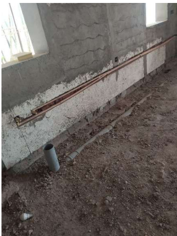
Fig 7: Termite activity is observed originating from the wooden pieces used as plumbing fixers. – Ground Floor
