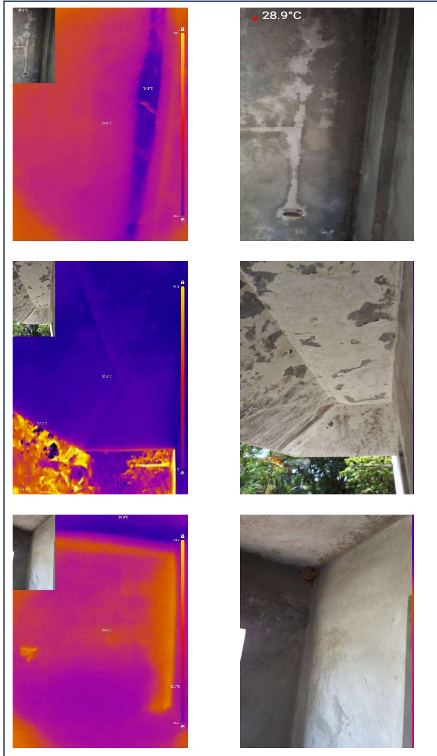
Fig 1: Dampness in a slab refers to the presence of moisture within the slab concrete. It occurs when water penetrates the slab due to improper waterproofing or the presence of cracks. – Grund floor
