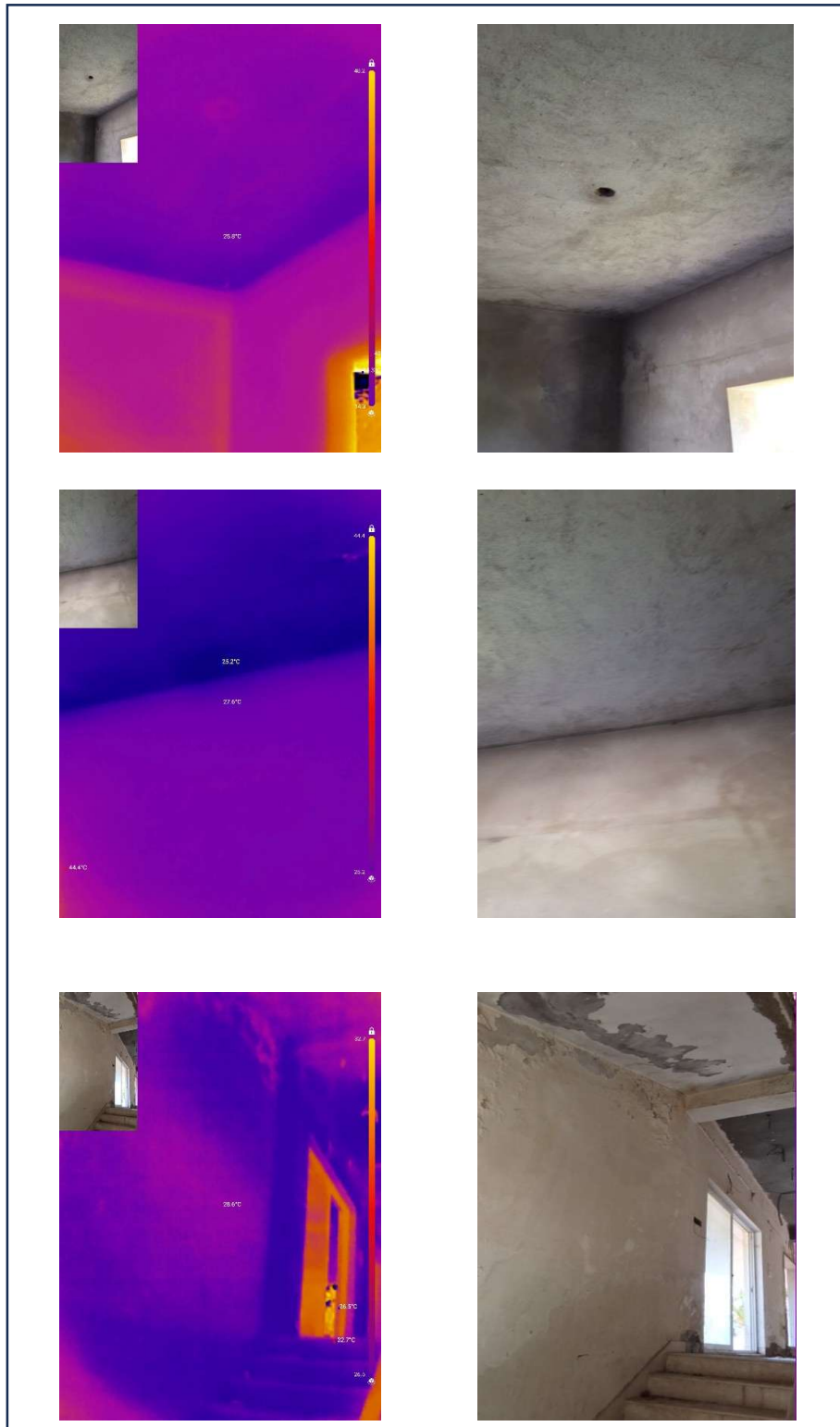
Fig 2: Dampness is observed transferring from the slab to the walls and staircase through the electrical conduit paths. – Ground floor
