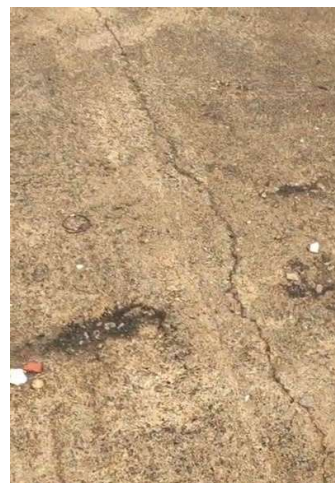
Fig 8: 20mm crack is observed on the 1 st floor front balcony for a length of about 25ft which lead to progressive deterioration of slab
