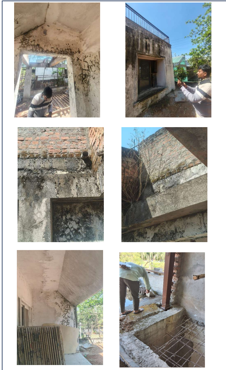
Fig 9:1. Water leakage from the slab into the walls, caused by improper compaction of concrete and absence of waterproofing on the slab, has deteriorated up to Stage-3 . due to improper maintenance. 2. Structure being unused and non-maintained, plantation observed on the structural elements.
