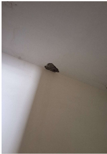
Fig 11: Debonding of the slab has occurred, leading to Stage-3 deterioration . – 1 ST floor
