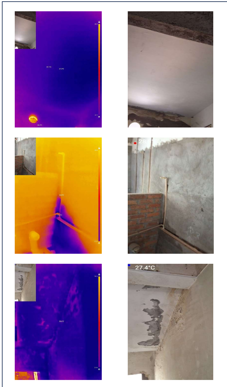
Fig 3: Dampness in the walls and slab is observed due to improper slope for water drainage, resulting in water stagnation and subsequent seepage into the slab. – Ground floor
